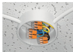
Lighting distribution in a ceiling canopy
